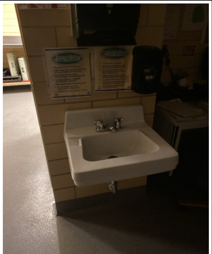
2/6/2024 - 1301-27 - Middle School - Kitchen- Handwashing Sink
