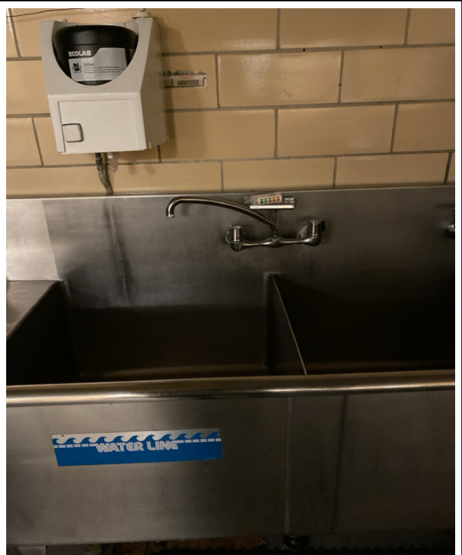
2/6/2024 - 1301-25 - Middle School - Kitchen- Three Bay Sink-Left
